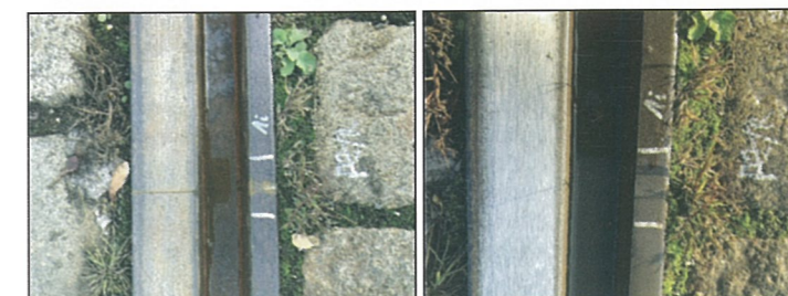
Fig. 4: A section of rail before (left) and after (right) oscillating rail grinding
