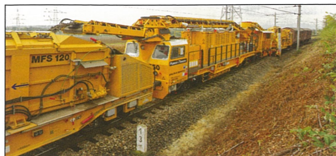
Fig. 6: Following in the footsteps of the RM 80 – the RM 85-750 MFS, featuring one ballast excavation chain and one screening unit
