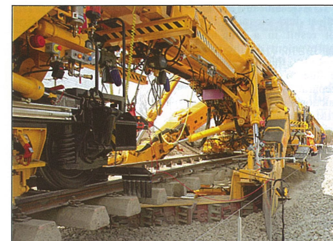
Fig. 10: RPM RS 900 formation rehabilitation machine with two ballast excavation chains and integrated ballast recycling – can work as a stand-alone ballast cleaning machine (picture also shows FPL insertion)
