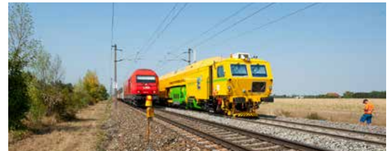
E 3 on track since 2015: the first development carrier was an Dynamic Tamping Express 09-4X E 3
