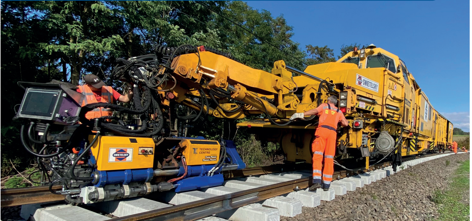
The Plasser FlashWelder was trialled in regular service by Swietelsky, mounted on a rail-bound carrier vehicle.
